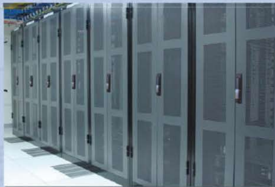
Access control at the server cabinets
